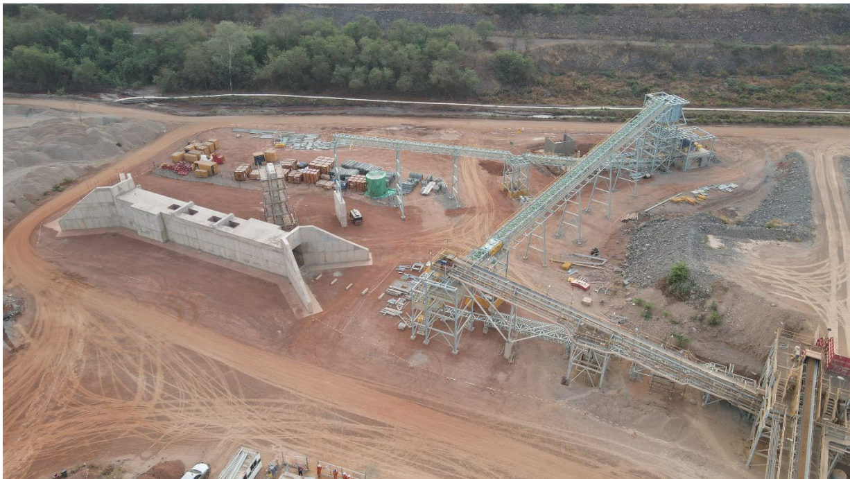
Figure 11: Secondary crusher and sulphide stockpile feed conveyor areas are 50% and 30% complete respectively
