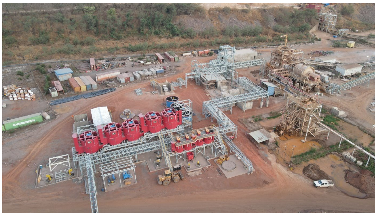
Figure 10: Ball mill and flotation areas in March under construction. The flotation circuit is now 86% complete, while the ball mill areas is 35% complete
