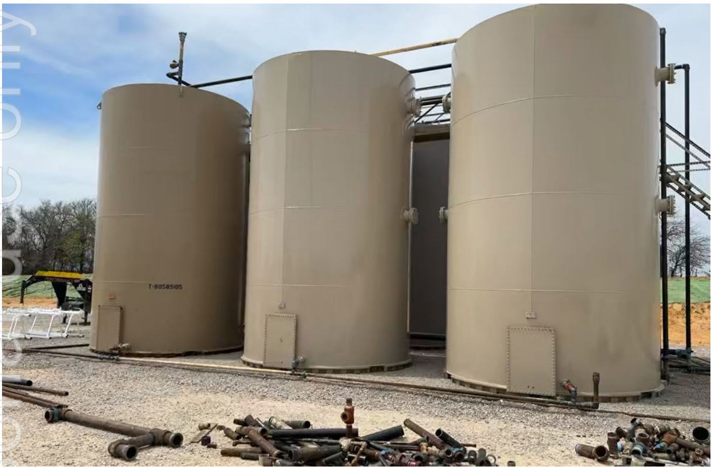
Figure 1. Oil storage tanks have been delivered to the Bruins Well site in the Company's SWISH Play as construction of permanent production facilities get underway.
