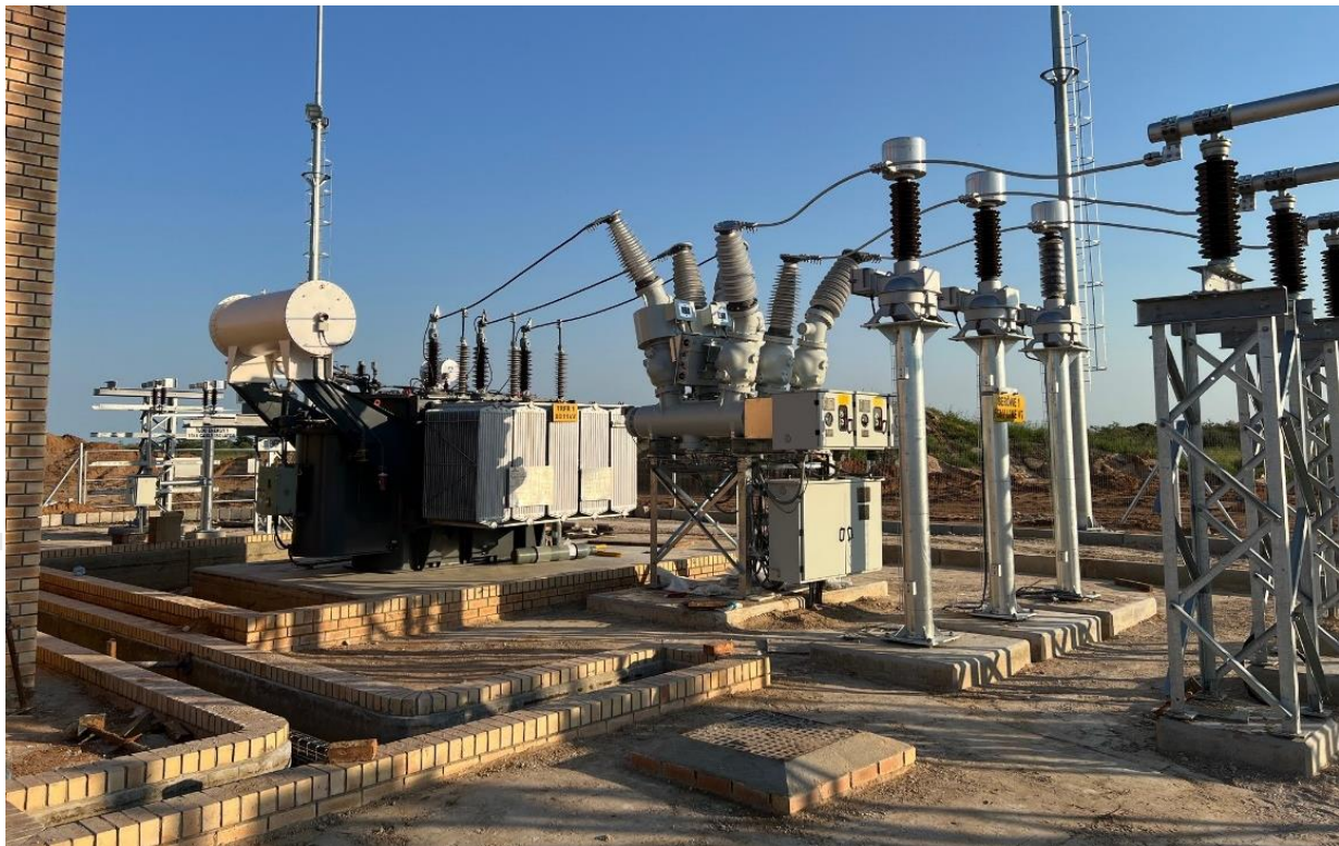
Lesedi Substation – Q1 2025
