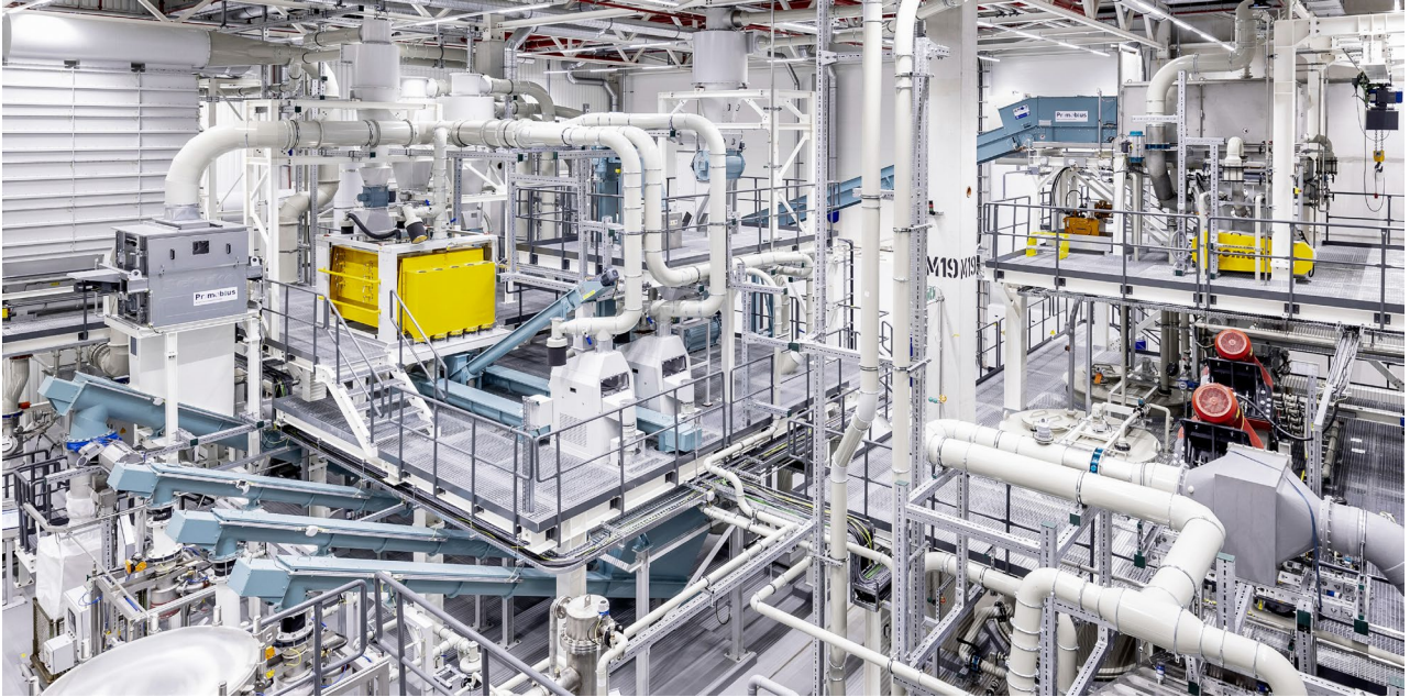
Figure 1 – Part of the Shredding and Beneficiation circuit installed by Primobius at Kuppenheim
