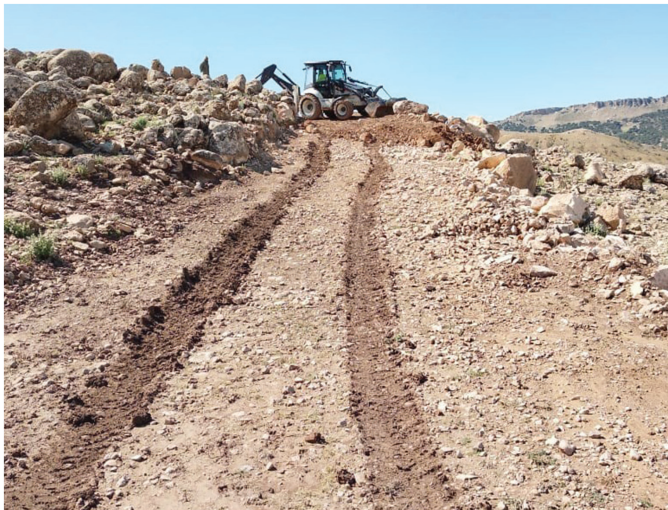
Access roads being prepared for the drill rig at Gasaat (GS prospect).
