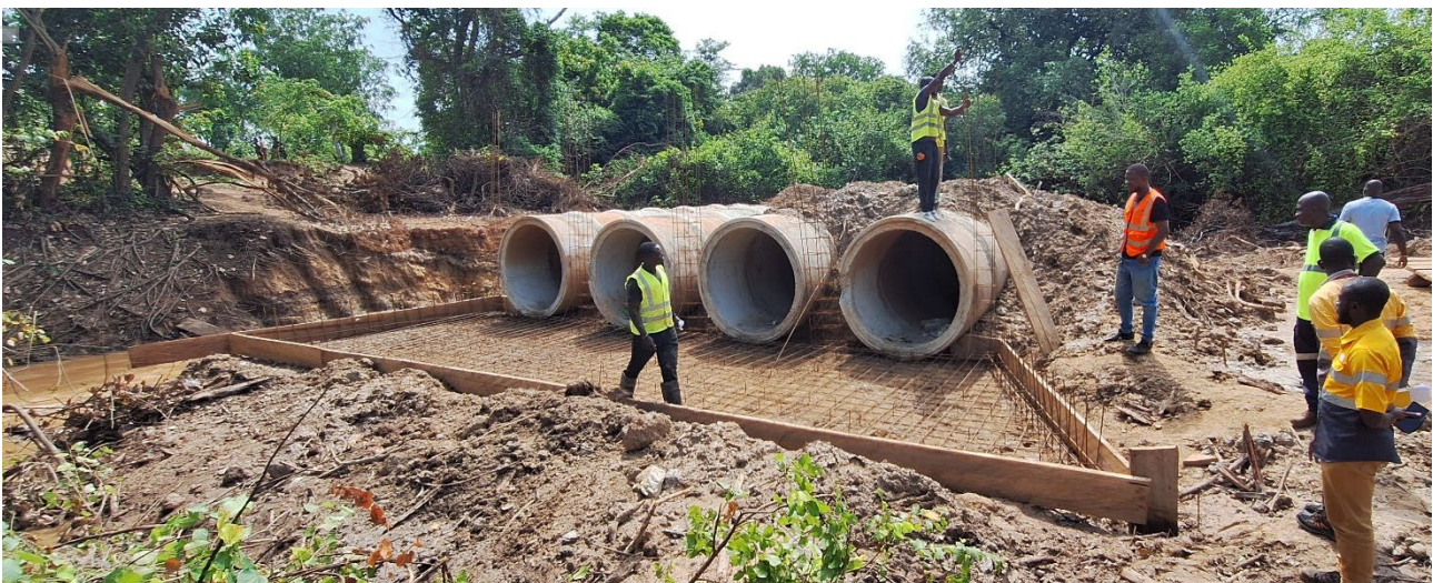
Figure 7: Construction in progress of a bridge between Napié's two existing gold deposits
