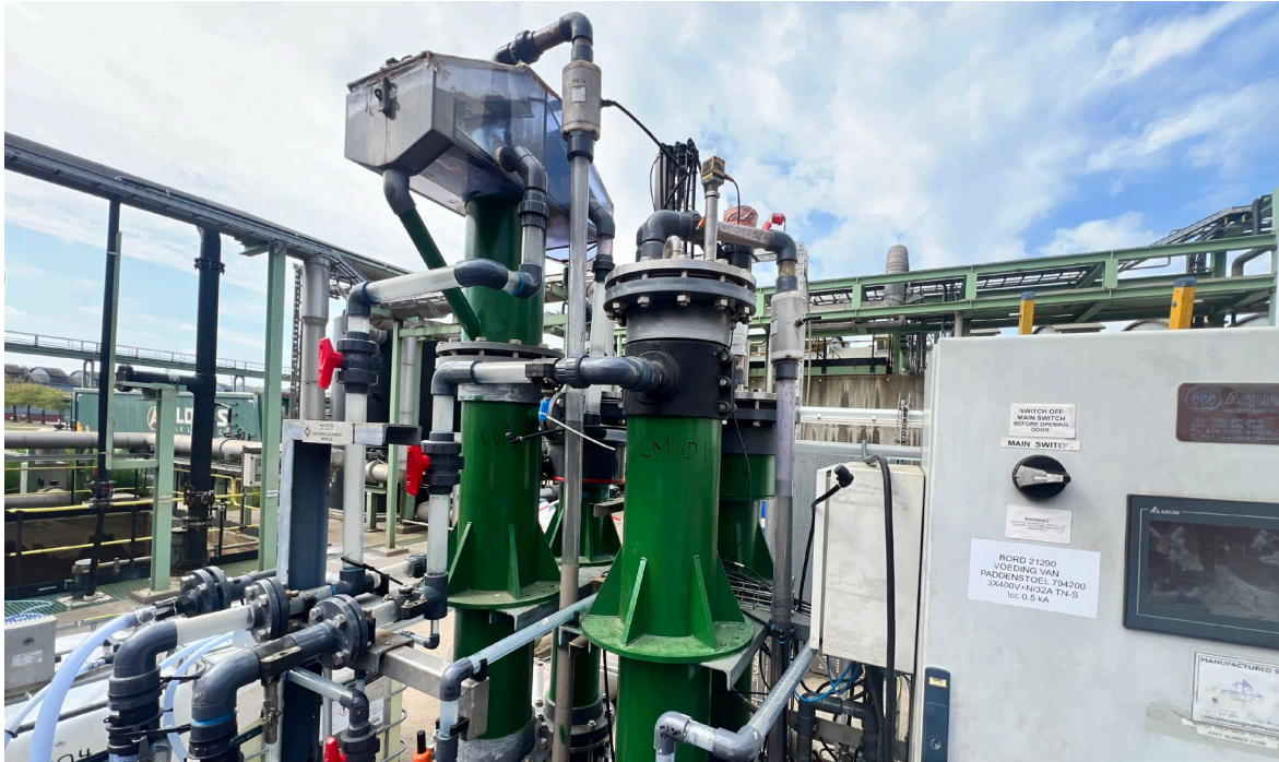
Clean TeQ's DESALX ® pilot plant successfully removed sulphate and selenium from Nyrstar smelter wastewater
