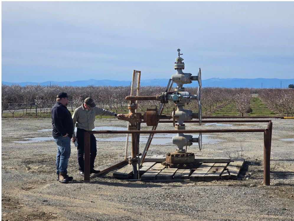
Figure 1 The Company's operated Dempsey 1-15 well with field personnel located in close proximity to the Stoney Creek Master Meter Station
