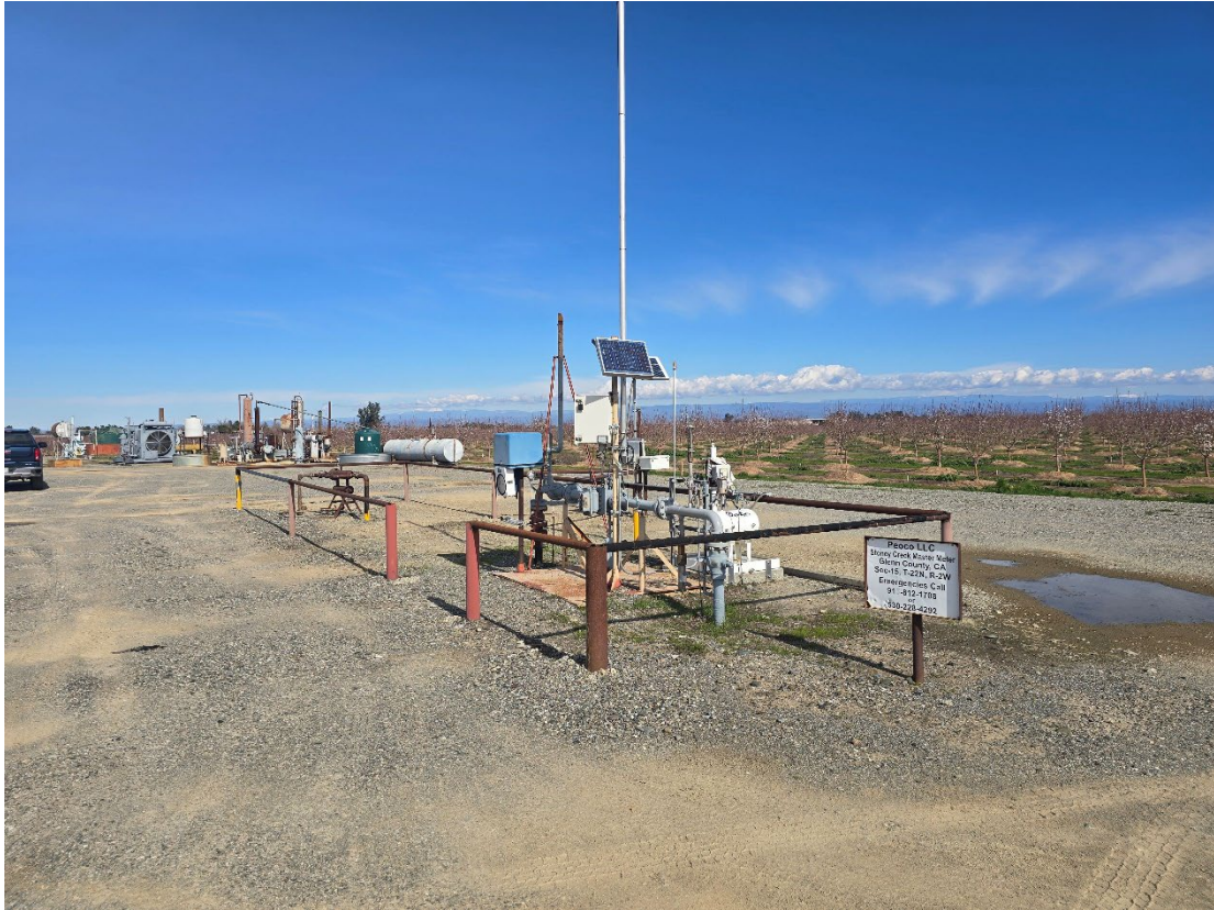
Figure 2 The Company's Stoney Creek Master Meter Station that measures production from Stoney Creek wells and Dempsey 1-15
