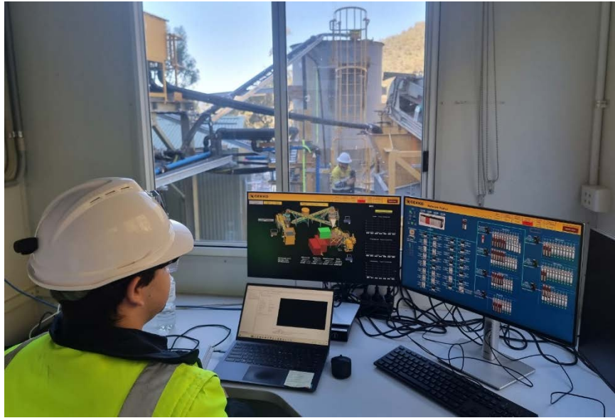
Figure 8: Automation programming technician testing the Reward gravity plant systems from control room
