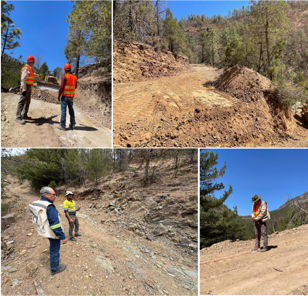
Figure 1. Composite image showing recent road repairs and drill pad construction in the Pertenencia area at Yoquivo.
