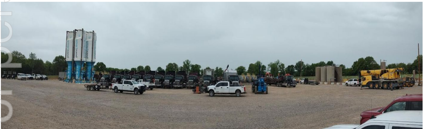
Figure 1: Completion crews and equipment mobilised on site at the Bruins Well. Infrastructure includes high-pressure pumps, sand silos, fluid storage units, and service vehicles ahead of 24-hour hydraulic fracturing operations.
