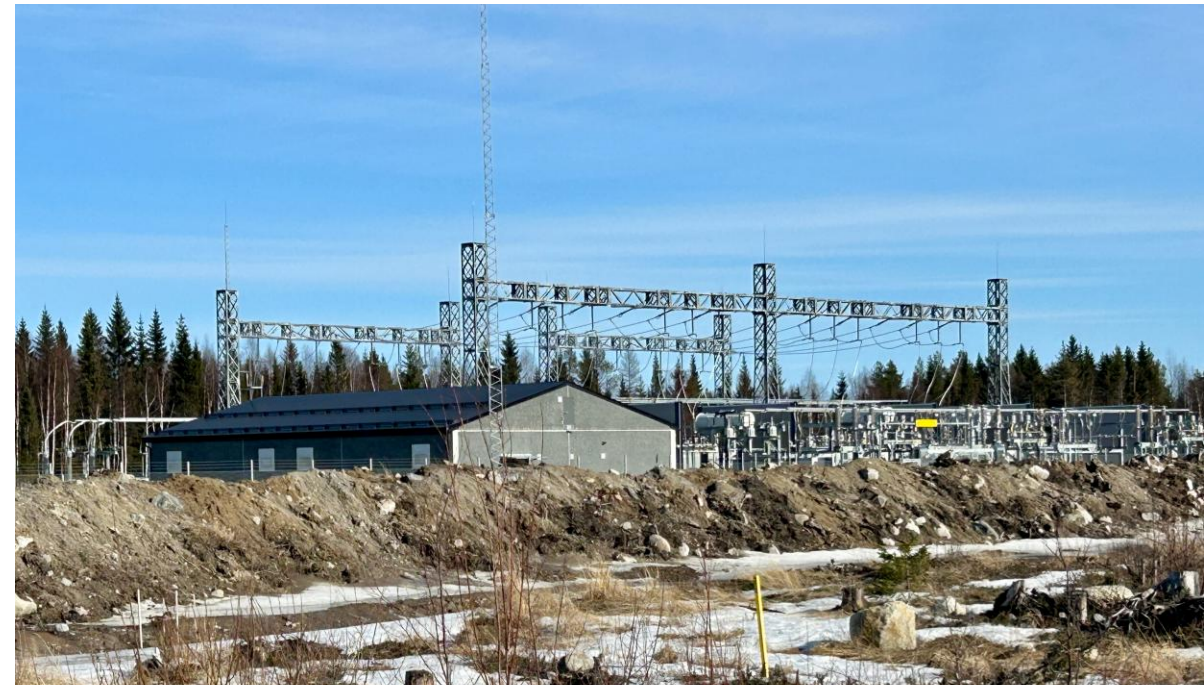
Electrical substation at Luleå Industrial Park, April 2025
