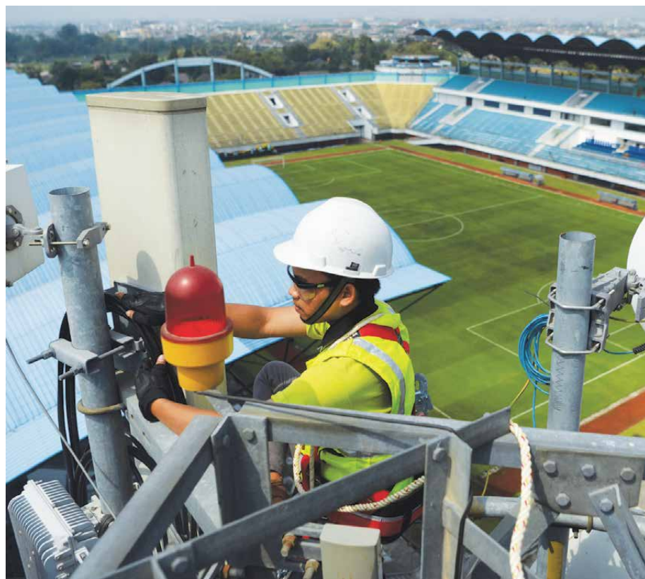
MAM manages an investment in Bersama Digital Infrastructure, which is pursuing telecommunication towers, fibre and data centre investment opportunities in Southeast Asia.
