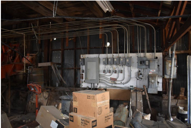
Photo 3. Electrical control board within the mill building.
