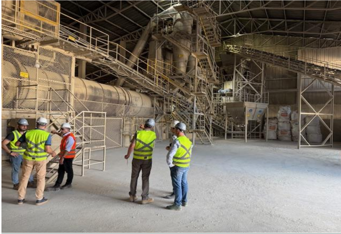
Rotary Dryer, Cacapava do Sul Processing Facility Asset to be leased by Aguia
