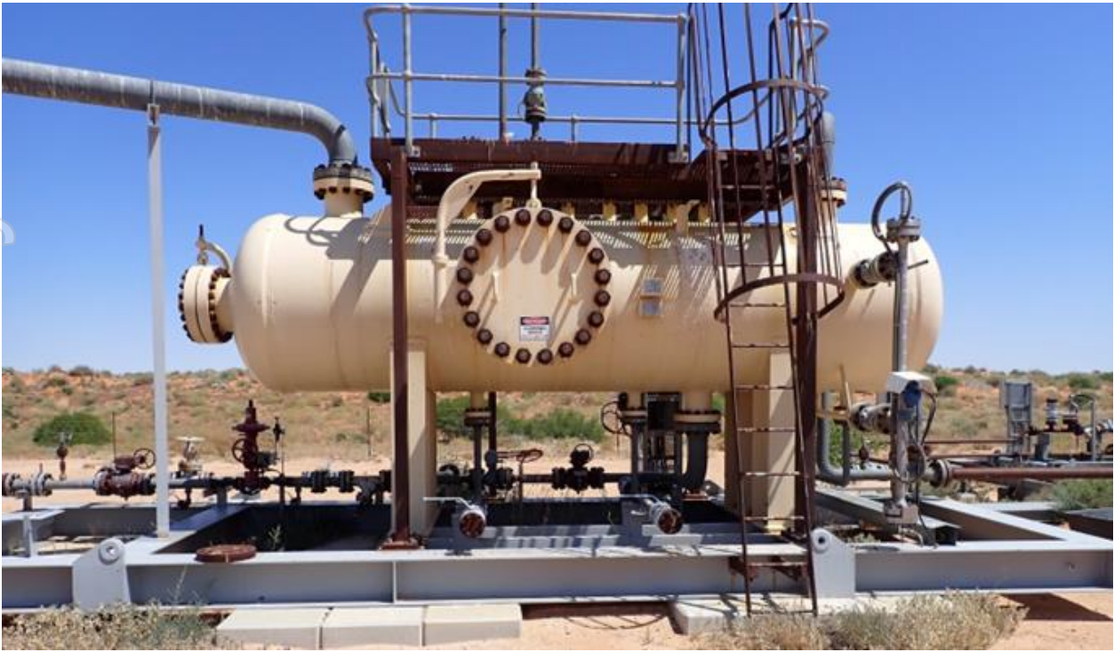
Figure 3: Gas/liquids separator in place at Vanessa facility.
