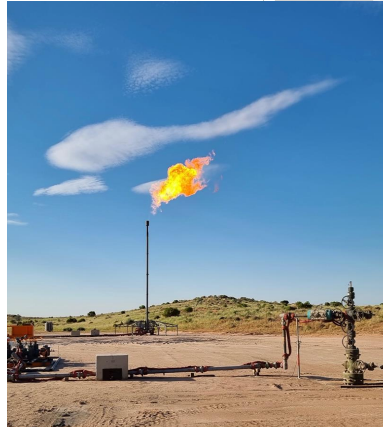
Figure 8: Gas flare from Kiwi-1 wellsite at 1.7 mmcf/d
