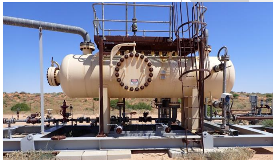
Figure 3: Gas/liquids separator in place at Vanessa facility
