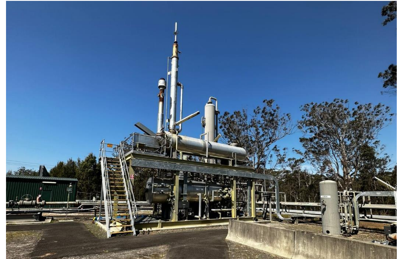
Carpentaria Gas Plant
