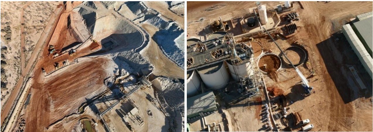
Figure 6: Stage 1 upgrade works underway with crusher excavation work (left) and new tank footings (right)
