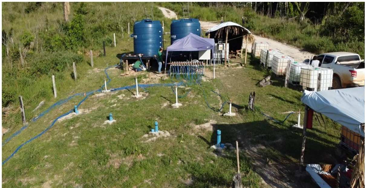
Figure 1. view of the water storage tanks piped to injection holes designed and drilled to optimise and test solution permeability.
