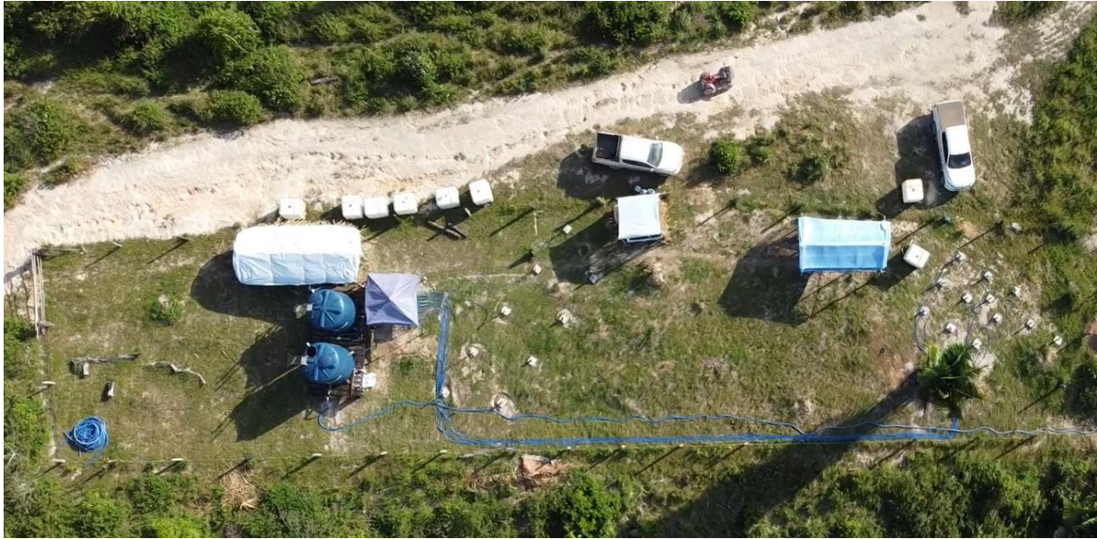
Figure 2. aerial view of the ISR setup, injection and extraction holes and associated infrastructure.
