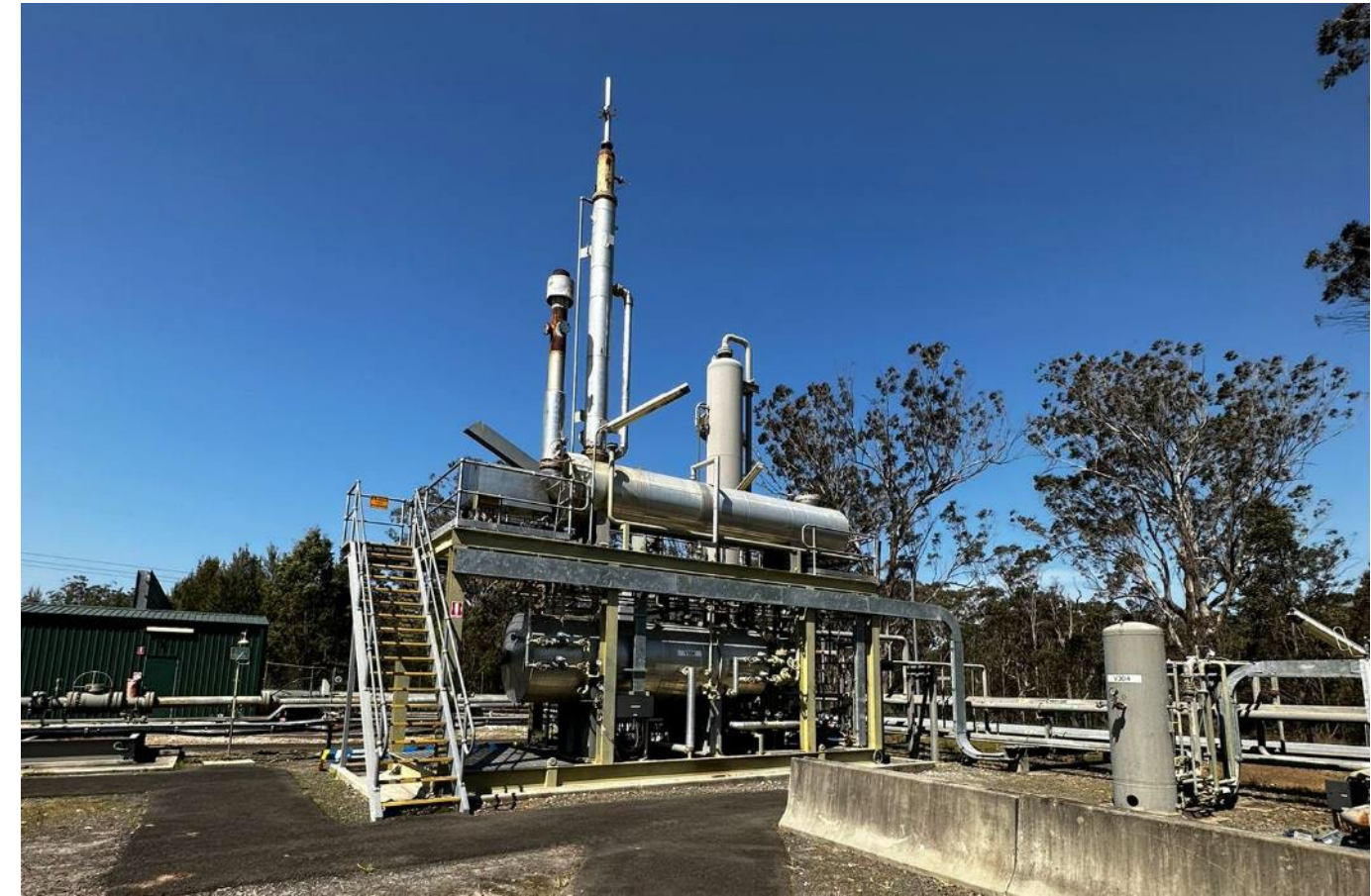
Carpentaria Gas Plant
