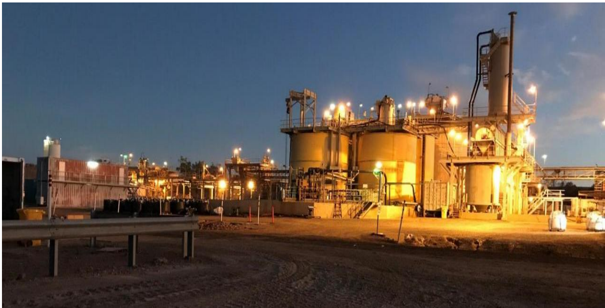
Figure A14: Existing CIL and Adsorption Tanks and Elution Column
