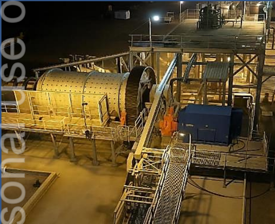
Figure: Existing 1800kW Ball Mill
