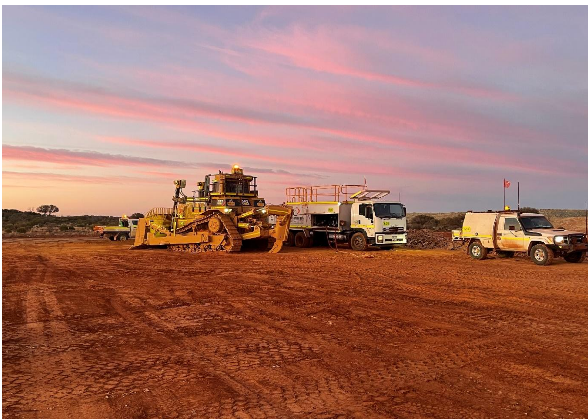
Plates 6 & 7 Installation of mine site offices (top) and first mining equipment arrival (bottom)
