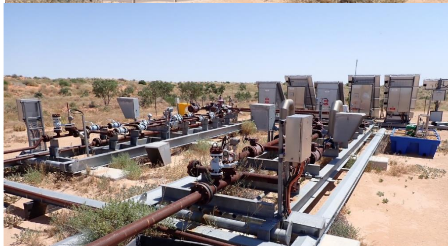
Figure 6: Gas/liquids separator in place at Vanessa facility Figure 7: Current infrastructure in place at the Vanessa facility
