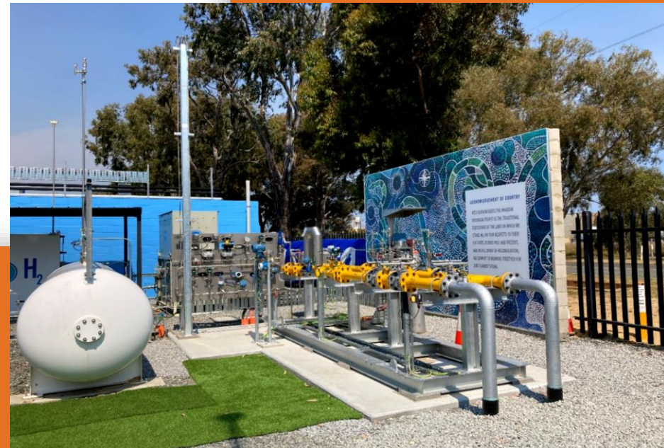
ATCO's fully commissioned H 2 Blending Station at Jandakot
