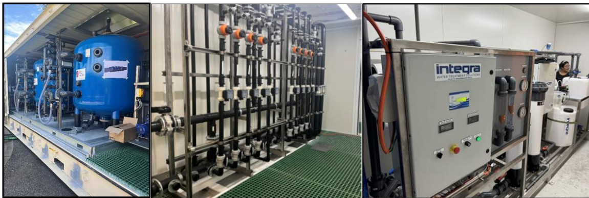
Fig 2 – Ion exchange module; Wellhouse (pipe room) module; Reverse Osmosis plant – all currently situated in Alligators Whyalla yard
