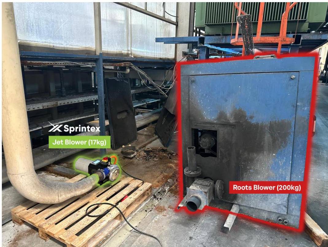
Sprintex Jet Blower 17kg (left) replaces Rotary Lobe (Roots Blower) 200kg (right) providing equal flow and pressure
