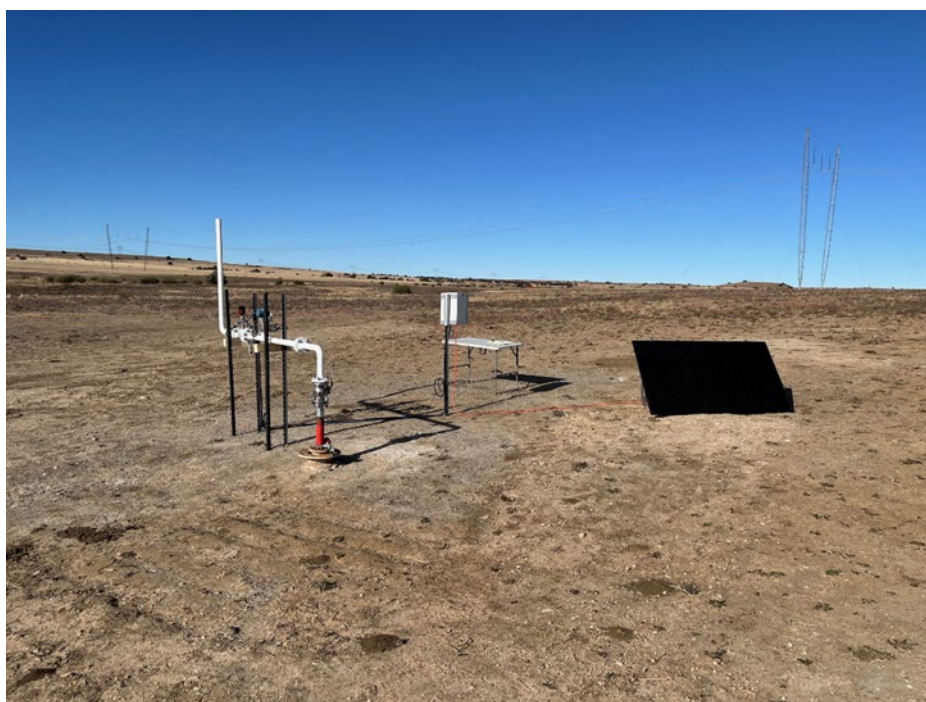
Testing Equipment at RBD03
