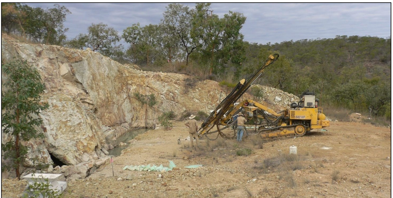
Figure 3: Shallow airtrack drilling beneath the 1991 trial pit at Francis Creek (from CR40465, 2005).
