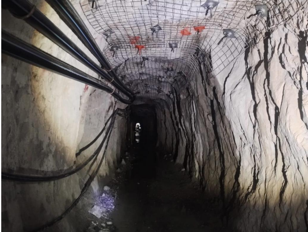
Figure 6 – Back height increased in the Amalgamated Adit to hang the High Voltage 11kV cables and services.
