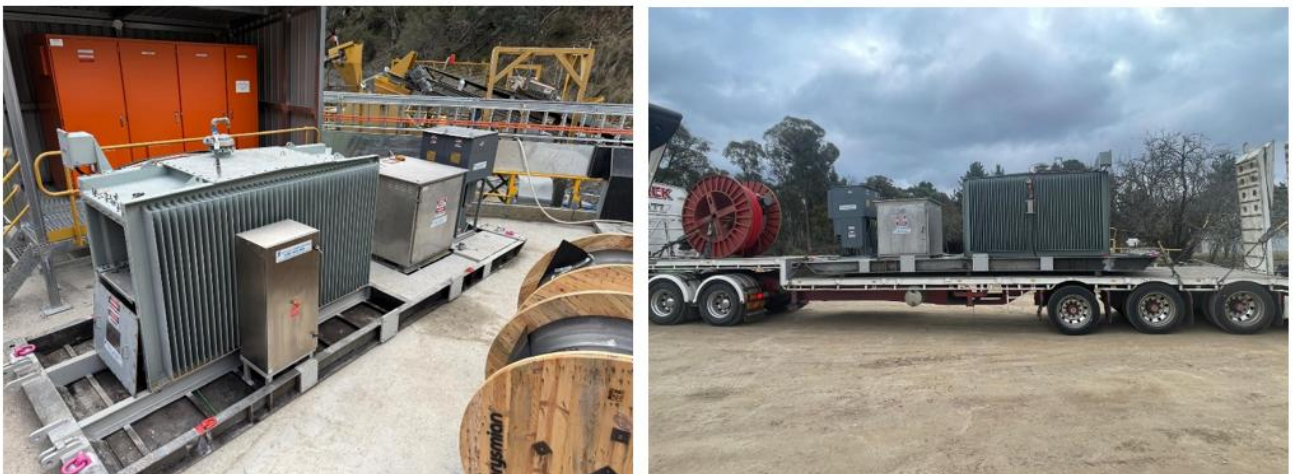
Figure 1 – High voltage (415V to 11kV) transformer installed next to power station at the Reward Gold plant
