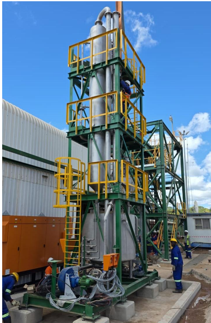
Figure 6: Placement of the new off-gas scrubber outside the drying and packaging building
