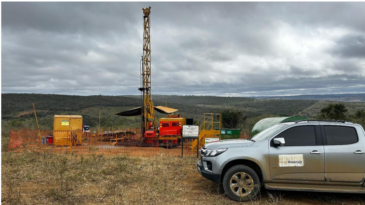
Figure 1. Diamond drill rig set up on IR-1 prospect ready to drill on 22 July 2025.
