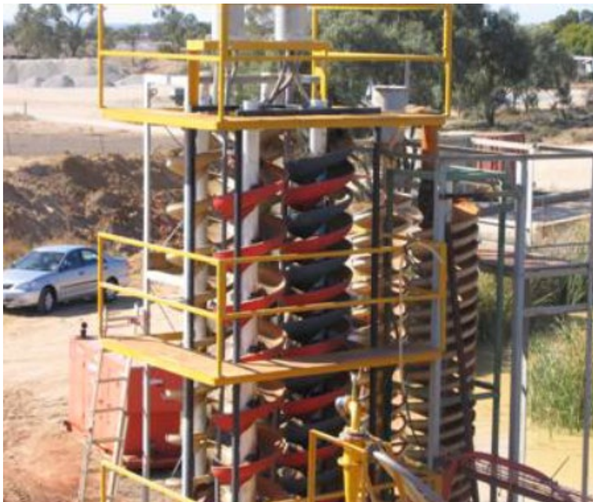
Figure 9 – Donald historical wet concentrator pilot plant in 2005
