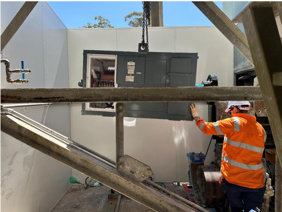
Figure 7 – DC mill motor installation
