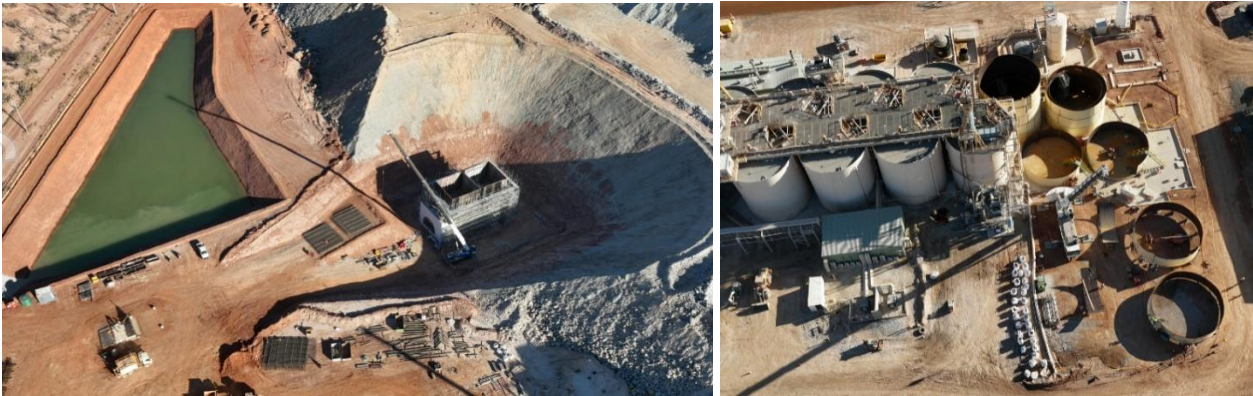
Figure 2: KoTH plant expansion project (crusher box cut excavation on left and tank erection progress on right)
