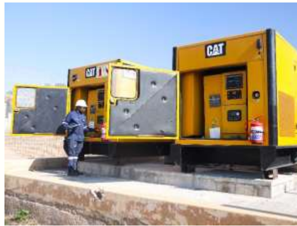
Temporary generators for the ramp-up phase
