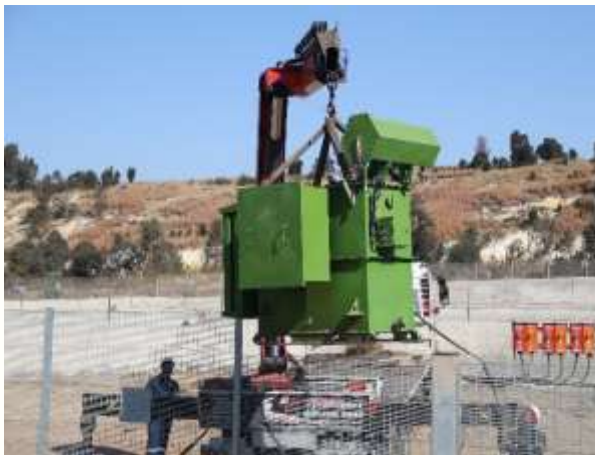
Serviced transformer delivered to site
