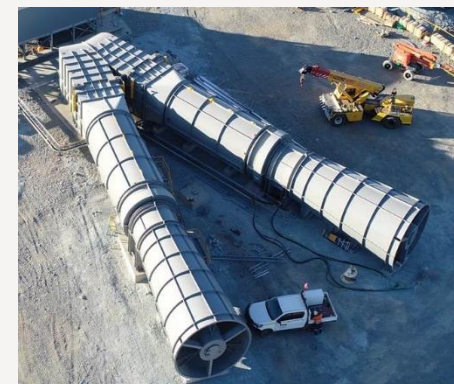
Underground primary ventilation
