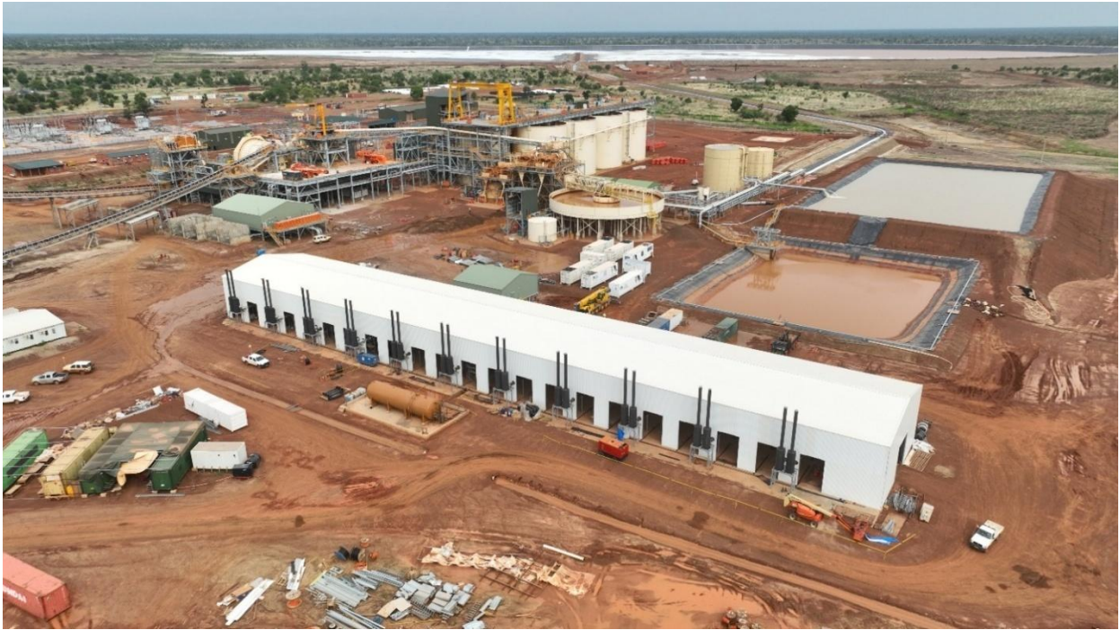
Kiaka Plant with Generator Shed in Foreground
