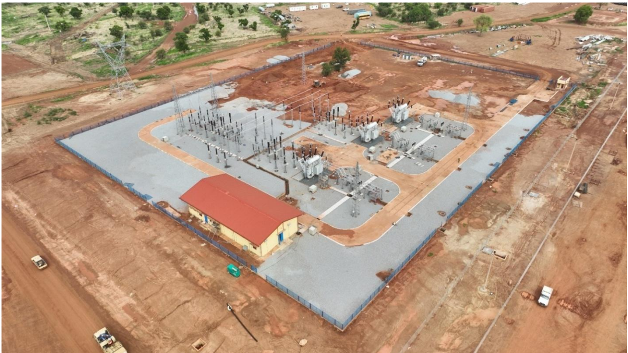
Kiaka Electric Power Substation
