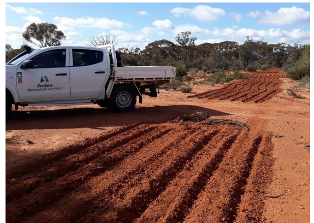
Figure 9: - left: Planned Goongarrie Hub in-pit tails disposal and rehabilitation strategy. Above- Showing scarification of disturbed areas, during rehabilitation of Goongarrie South drill sites.
