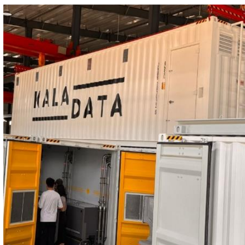
Data Centre Facility
