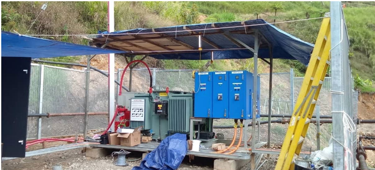
Photo 5: Electrical installation at the main portal
