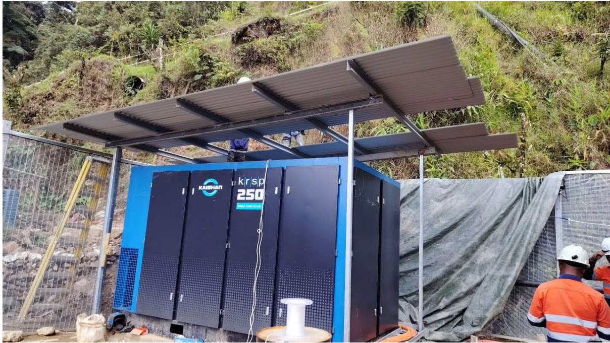
Photo 6: Main portal compressor
