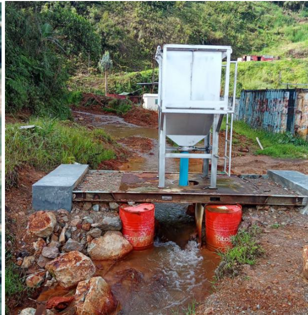
Photo 1: Lime Dosing Hoper
