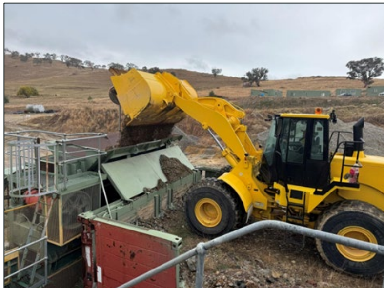
Figure 1: Loader tipping remnant high-grade ore to crushing circuit (GDM ASX Announcement 2 June 2025)
