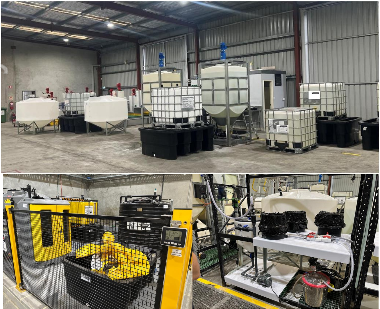
Figure 8. The HiPurA pilot plant: note the filtration units still in wrappers.
