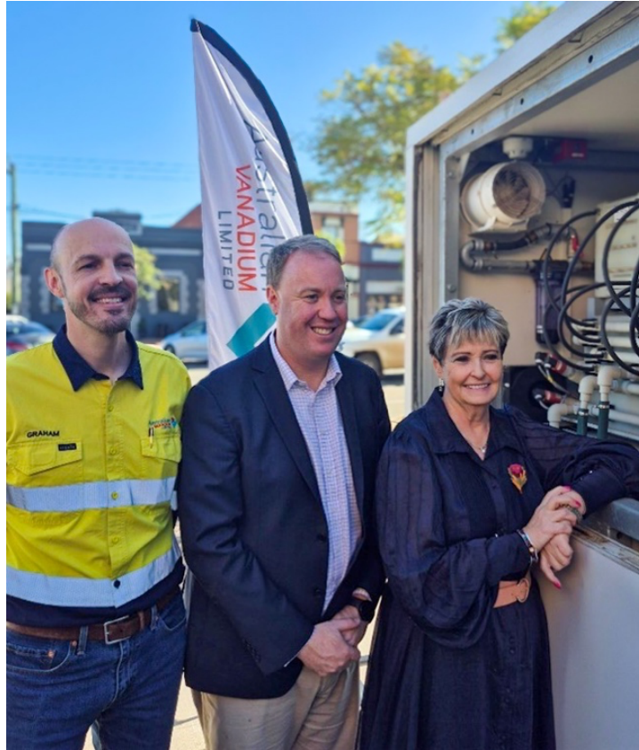
Figure 5 – VSUN Energy demonstration vanadium flow battery at Curtin University’s WA School of Mines Kalgoorlie Campus, with Hon David Michael Minister for Mines and Goldfields-Esperance, Ali Kent MLA Member for Kalgoorlie and Graham Arvidson CEO
