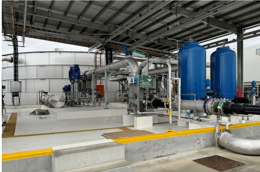
Townsville Water Recycling Facility to enter final stage of Performance Testing
