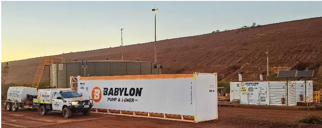
Remote power supply at iron ore mine site
