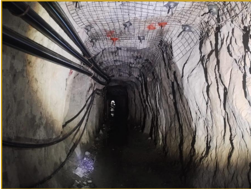
Figure 7 Backs height stripped meshed and bolted to give more clearance for equipment in the Amalgamated Adit.
