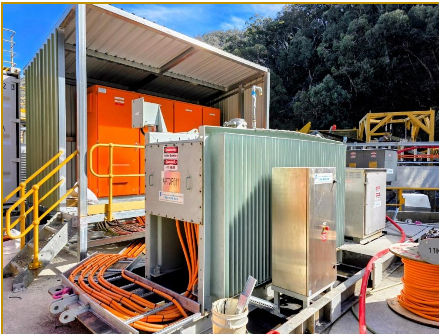
Figure 6 Installed 415 Volt to 11,000 volt transformer outside the Reward mine
