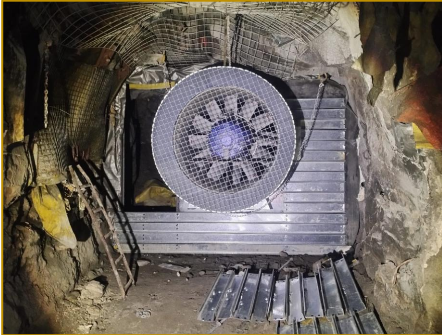
Figure 5 New Primary Fan installed ready for powering up with 1000v power
