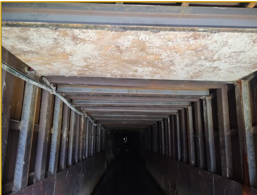
Figure 8 New steel sets installed to reinforce the Portal structure into the Reward Mine.
