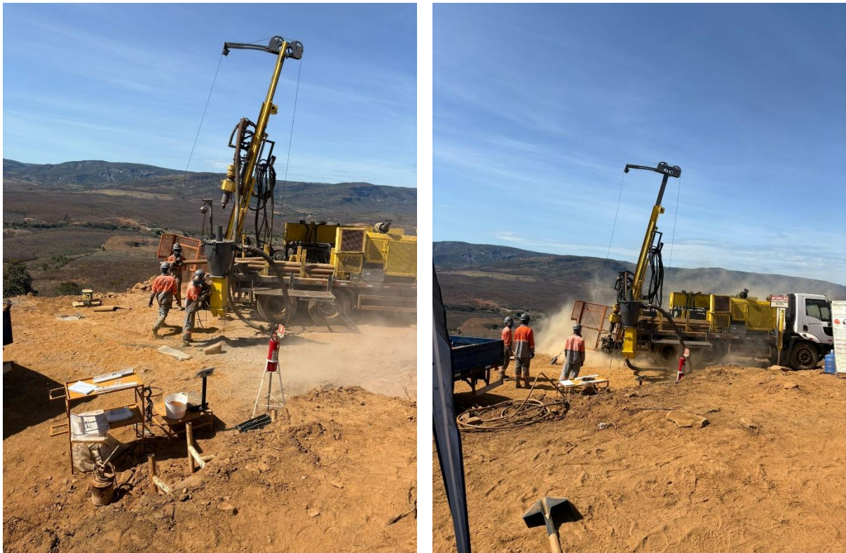
Figure 2: Image showing Reverse Circulation (RC) drilling underway at "Target 1" at the Igrejinha Lithium Project.
