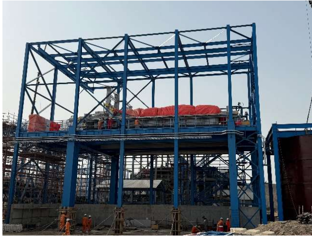
Image: New structure housing recently installed Tailing Filter Presses
